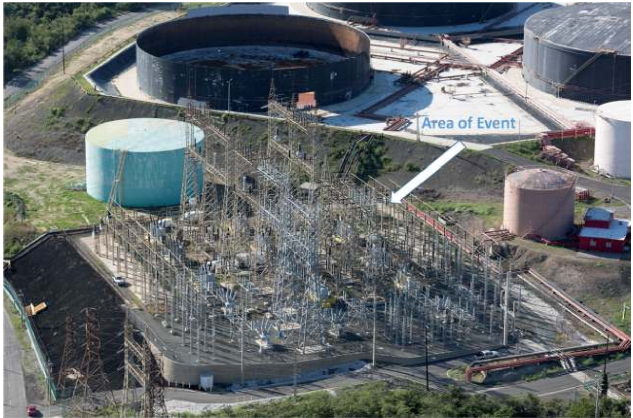
Figure 2: Costa Sur SP's 230 kV Switchyard (CB 0082 is in top right corner of photograph)
